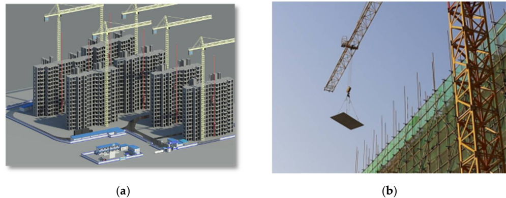
Figure 7. Construction site of the project. (a) BIM model of construction project; (b) On-site construction.
