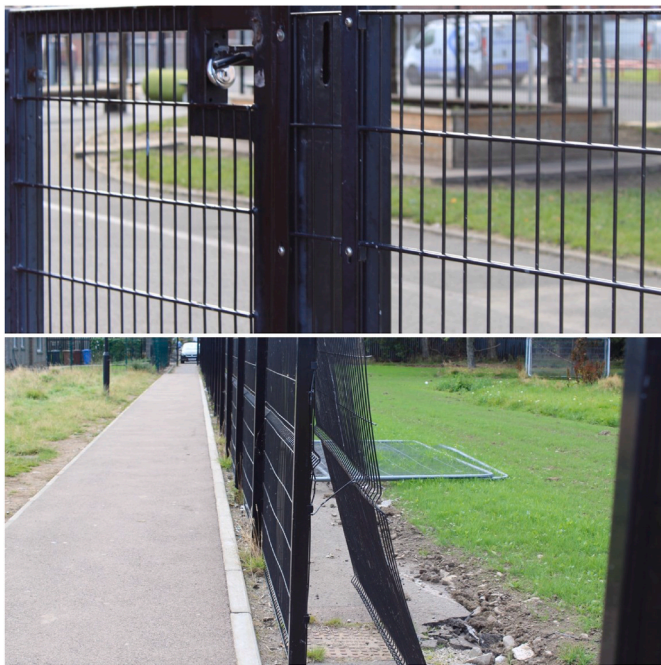
Fig. 2. a Secure fence around school. b Broken fence around school.
