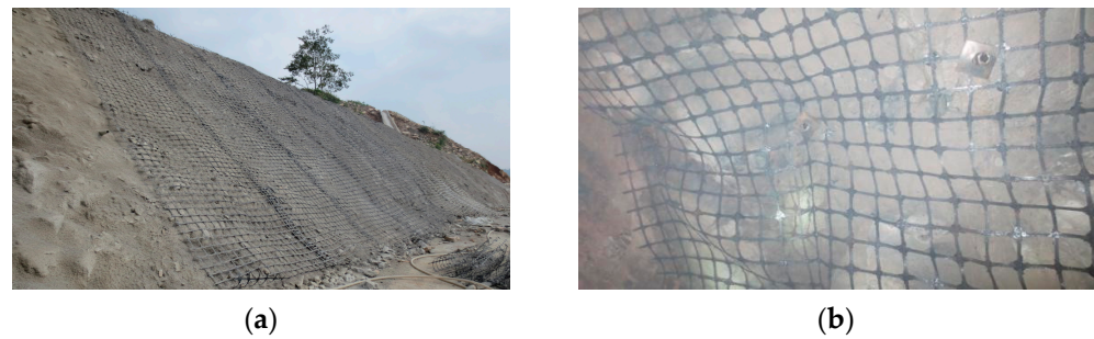
Figure 1. Engineering application of a steel–plastic compound geogrid: (a) slope support (b) roadway support.
