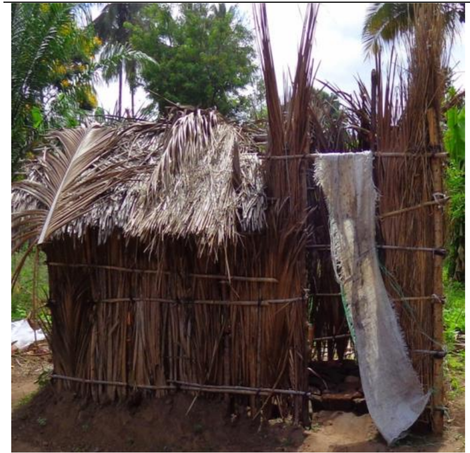
Fig 1. A pit latrine built with temporary materials and lacking door shutter in one of the study areas, Tanzania.
