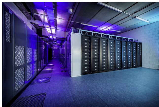
Fig. 2. Racks with part of the 2.8MWh energy storage system at the “Johan Cruyff Arena”. [Photo courtesy of Eaton].
