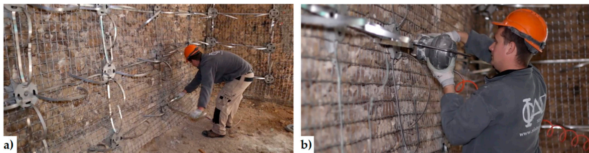
Figure 13. How to tie a masonry wall with the \Phi system: (a) housing of the ribbons on the internal face of the wall; (b) clamping of ribbons [54].
