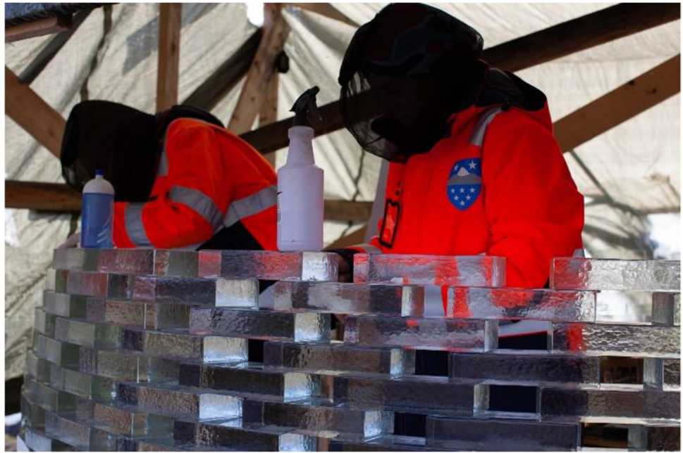
Fig. 21 The two TU Delft researchers bonding glass bricks on-site. Besides the adverse climate conditions, mosquitos proved to be an equal challenge in Greenland, deeming the use of mosquito nets necessary
