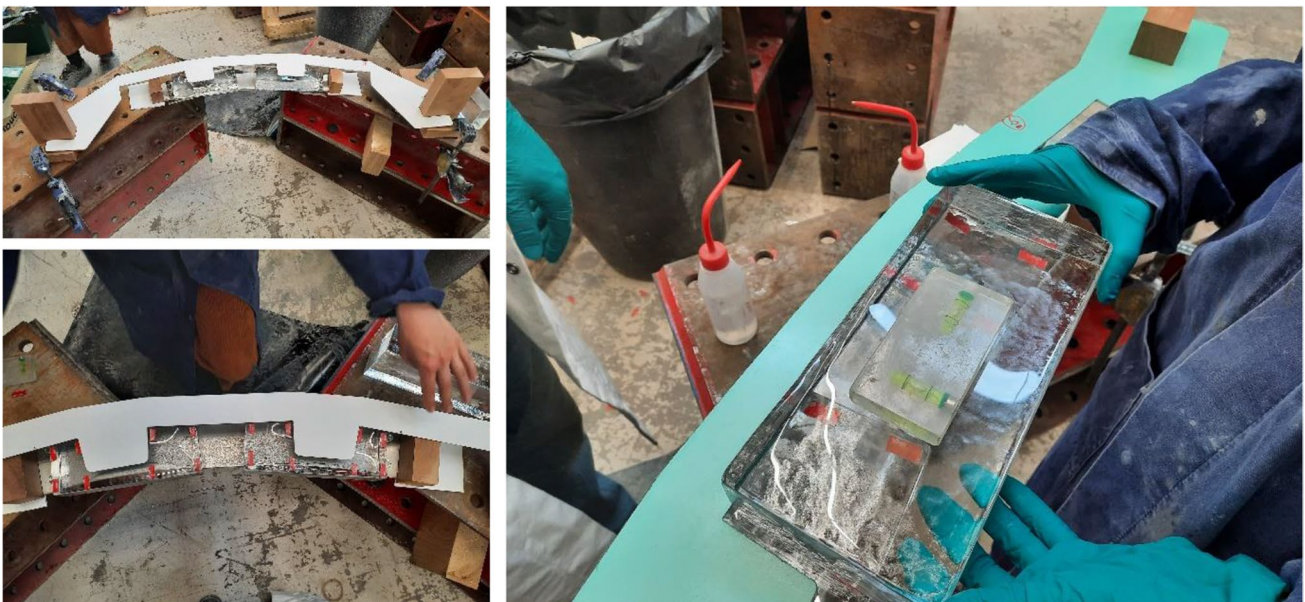
Fig. 16 Templates and wooden guides used to indicate the correct position of the glass bricks (left). Levelling of the glass brick with the help of a water-level and additional 0.5 mm double-sided tape stickers (right)
