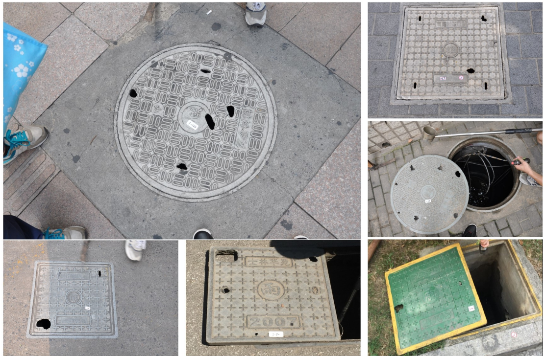
Fig 10. Examples of aging and broken MCs covers made of plastic composite.
