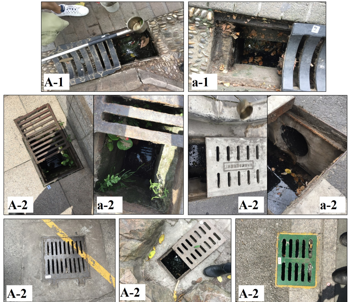
Fig 3. Examples of CBs with flat grates, including those (A-1) connected with surface gutters, and those (A-2) that are independent; (a-1,2) the insides of CB chambers.
