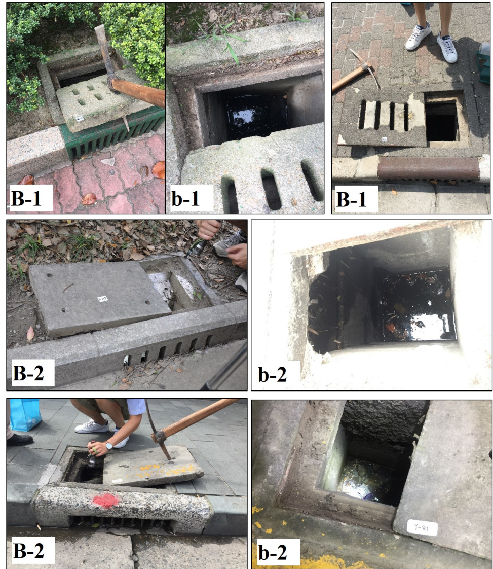
Fig 4. Examples of CBs with vertical grates: including those (B-1) with unsealed lids, and those (B-2) with sealed lids; (b-1,2) the insides of CB chambers.
