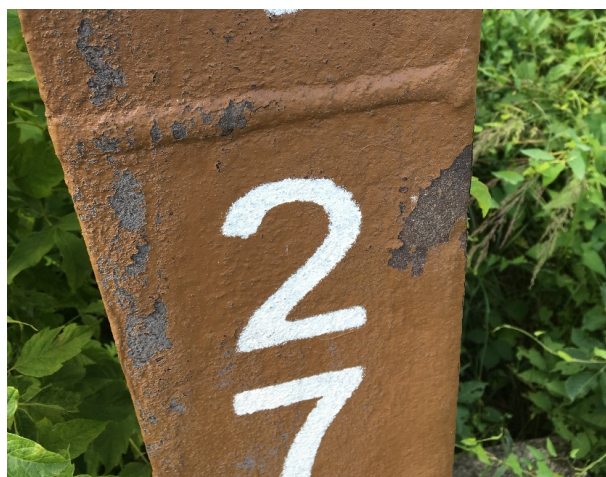
Figure 17. Failure of a paint system applied to a poorly prepared surface (the original protective layer of corrosion products remains under the peeling paint).
