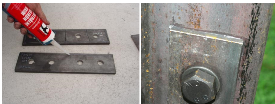
Figure 8. Application of silicone sealant ((left) application of sealant to the splices; (right) sealant smoothed around the perimeter of the splice).
