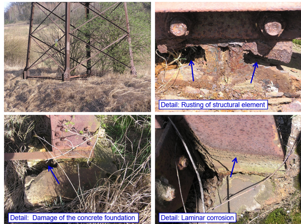
Figure 24. Selected examples of corrosion damage in the anchorage area of transmission towers.
