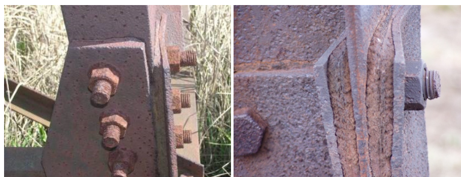
Figure 1. Crevice corrosion in the bolted joint of the leg member.
