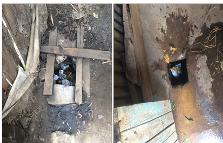
Fig. 2 Solid waste disposal into the pit latrine (a-book pages & papers, b-diapers)
