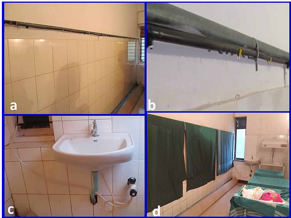
FIGURE 2: Humidifying system in the incubator room
