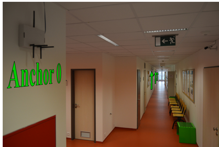
Figure 4. The installed anchors [12]. The photo is taken from the marked position (red camera in Figure 3), Anchor 0 and green arrows indicate anchors' position.
