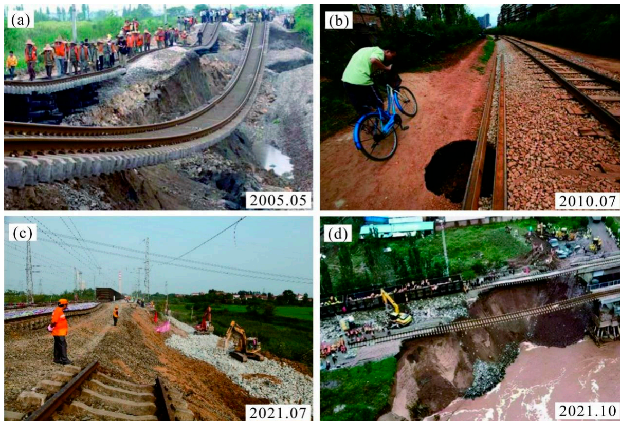
Figure 1. Typical high-speed railway foundation settlement disasters in China: (a) Xiaoyong railway collapse disaster; (b) Kunming railway collapse disaster; (c) Longhai railway collapse disaster; (d) South Tongpu railway collapse disaster.
