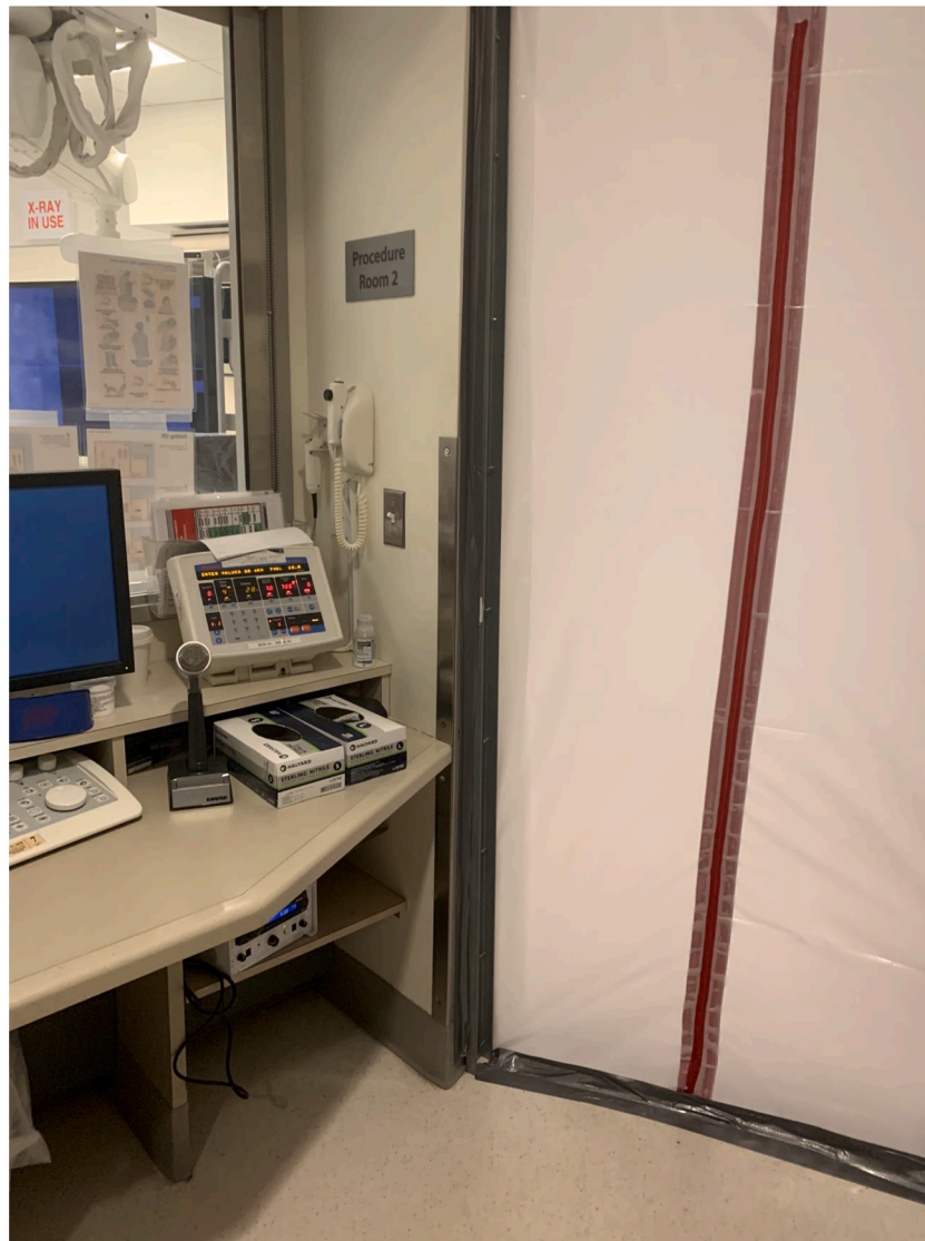
Fig. 3. Control Room Zipper Door “Bowing” into Anteroom –indicating positive pressure in control room
