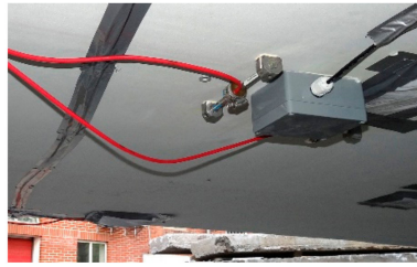
Figure 7. VWSG sensor fixed to the bridge.
