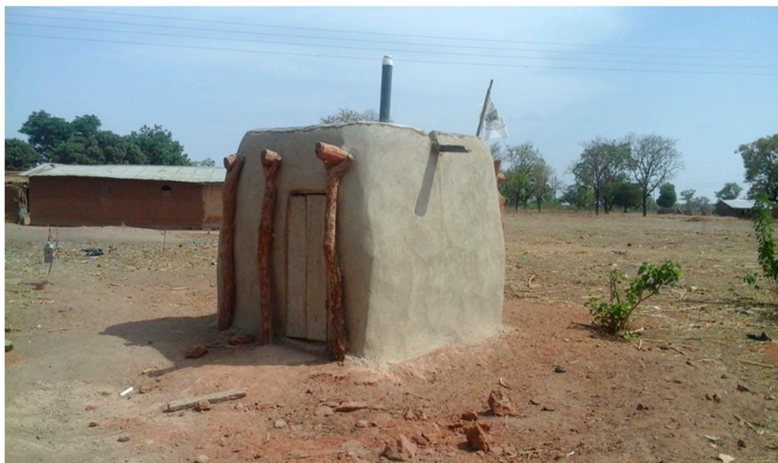
Figure 5. Pit is dug, superstructure constructed, latrines is roofed, latrine has door and a ventpipe.
