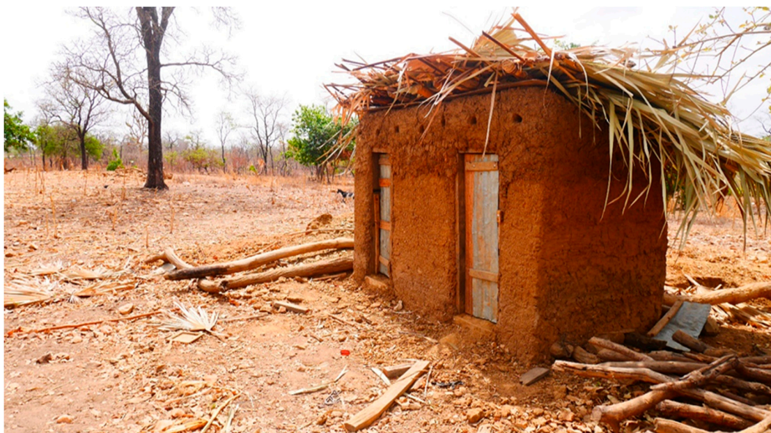
Figure 4. Pit is dug, superstructure constructed, latrine is roofed and door is fitted.
