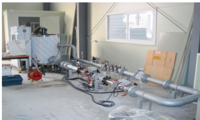
Figure 11. Pilot plant system.
