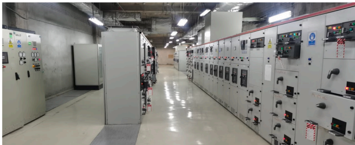
Fig. 1. High voltage power station of the power plant.
