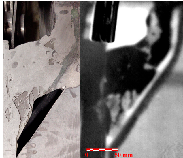
Figure 21. Comparison of NDE findings at the location of the flap lever seating ( right ) with the actual condition of the adhesive joint ( left ).
