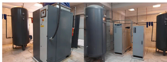
Fig. 1. Picture of the central oxygen concentrator unit in the hospital.
