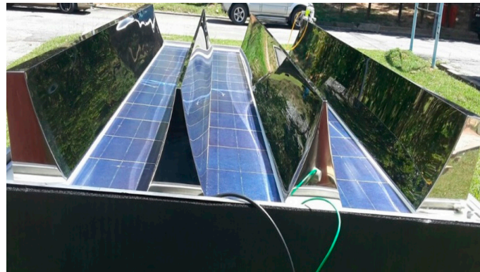
Figure 1. Photograph of the photovoltaic compound parabolic concentrator (PVT-CPC) collector.
