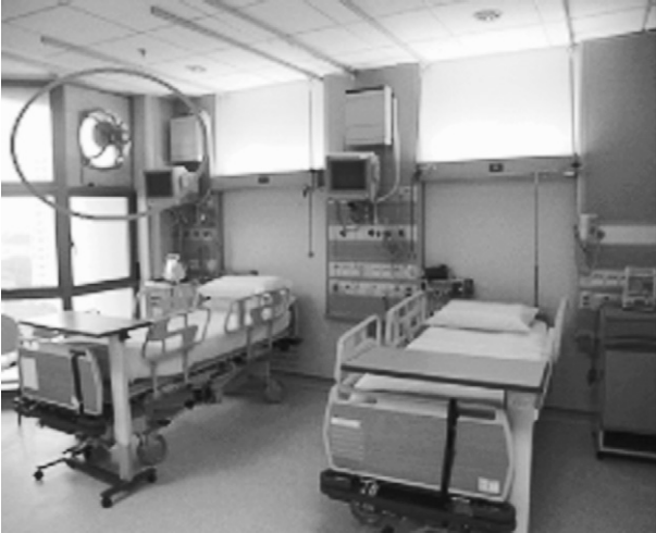
Figure 1. Installation of a window-mounted exhaust fan in a hospital ward. (Reprinted by permission from Annals, Academy of Science Singapore: Dessmon YH Tai, SARS: How to Manage Future Outbreaks? Annals, Academy of Medicine , 2006; 35: 368–373.)
