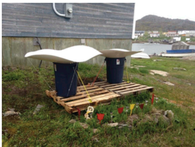
Figure 1. Example of a DRWH unit installed in the community.
